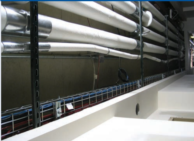
PHOTO 2 Plastic pipe bowing due to expansion.
